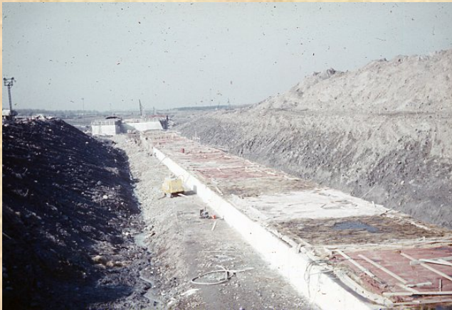
Bottom of Lock
